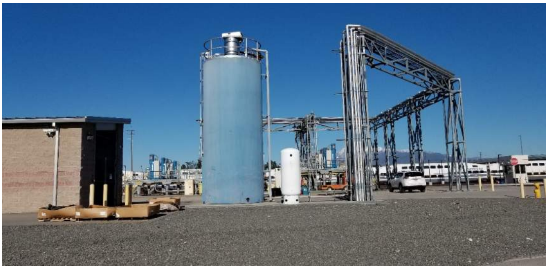
FIGURE 1-H. OVERHEAD PIPED SANDING FROM SAND SILO
