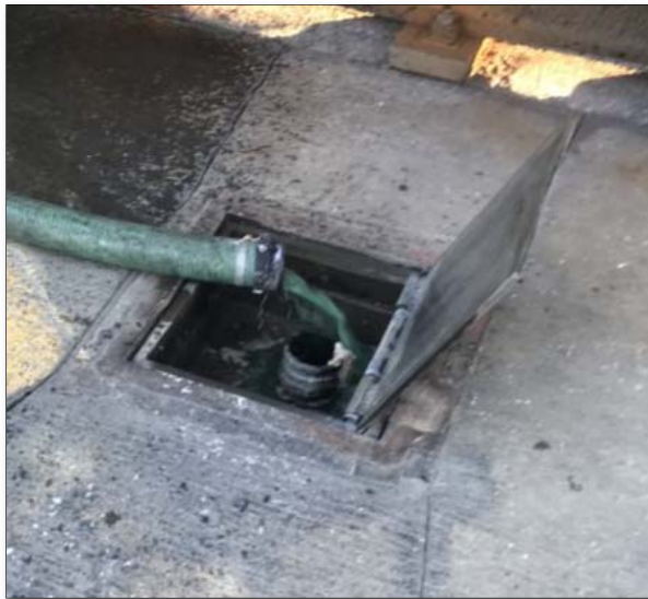
Ex. 16- Improper Connection
