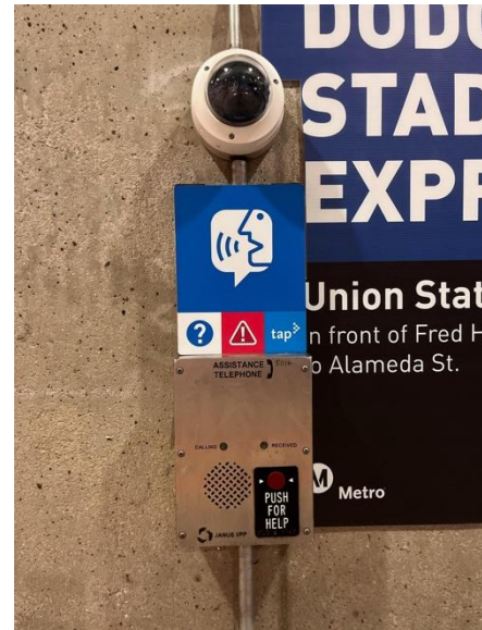
Figure 1 - Metro Rail Gate Telephone (G-Tel)
