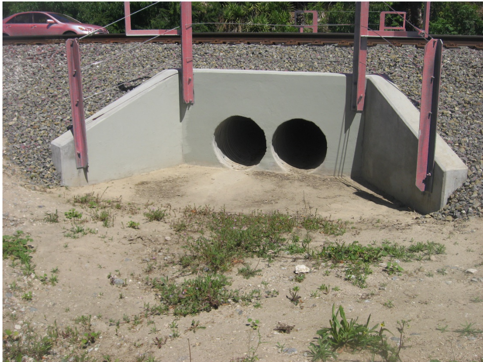
Photograph 10: Outlet of existing double culvert MP 436.56 passing beneath the rail looking north. No OHWM, bed or bank present (4/21/2020).
