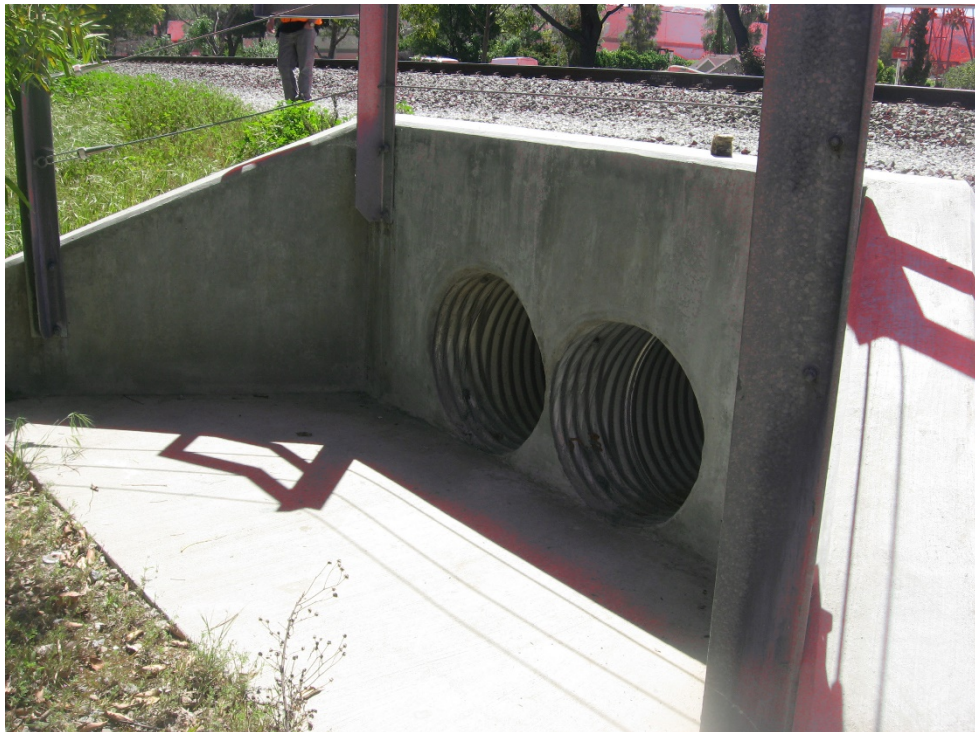
Photograph 8: Inlet of existing double culvert MP 436.56 passing beneath the rail looking southeast. No OHWM, bed or bank present. Based on historic topographic maps, this location did not support a defined drainage (4/21/2020).
