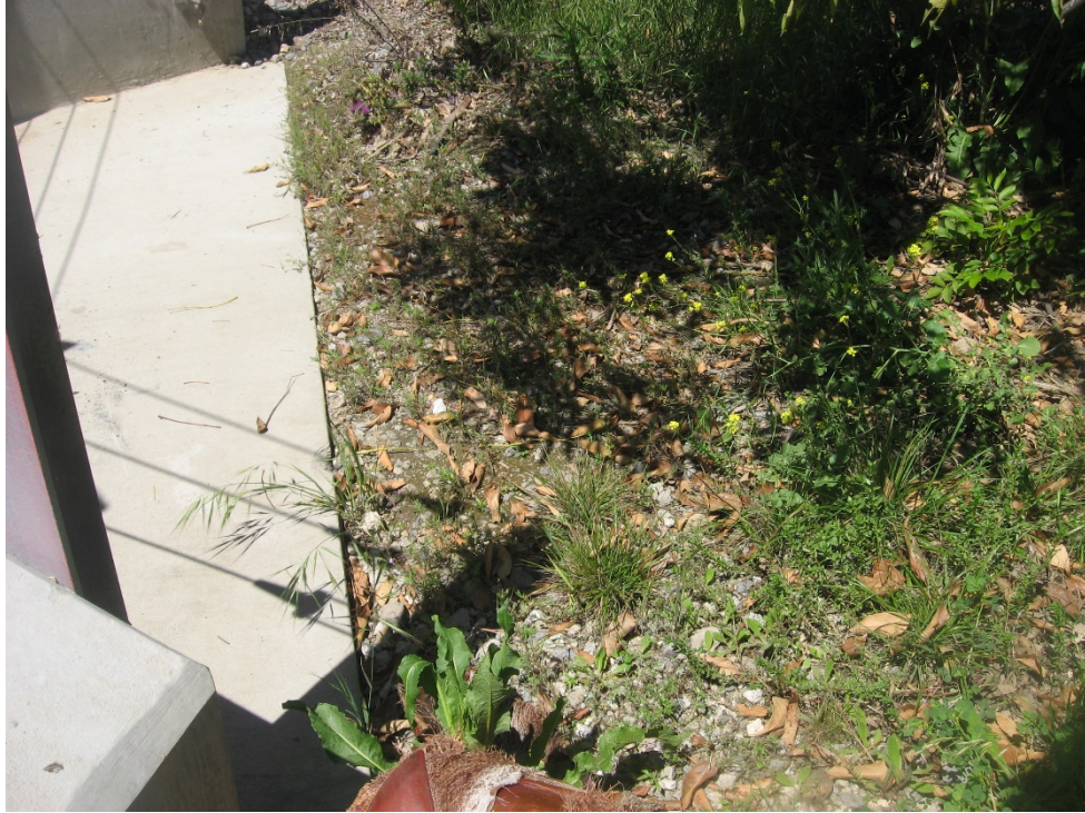
Photograph 9: Close-up view of culvert MP 436.56 inlet. No OHWM, bed or bank present (4/21/2020).
