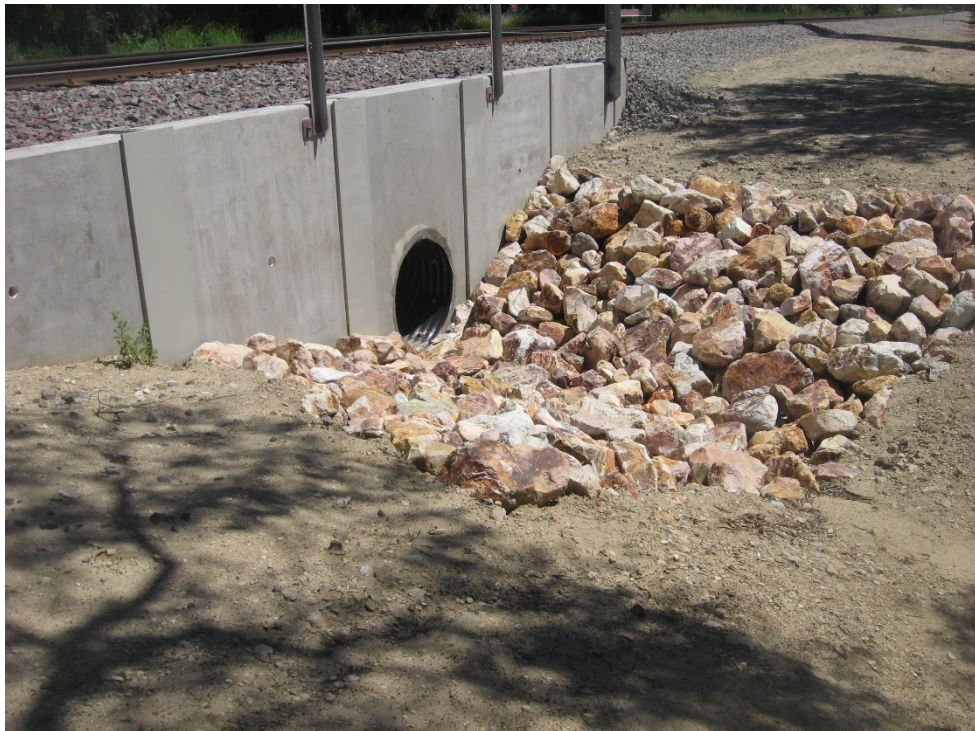
Photograph 14: Outlet of existing culvert MP 436.96 passing beneath the rail looking northeast. No OHWM, bed or bank present (4/21/2020).
