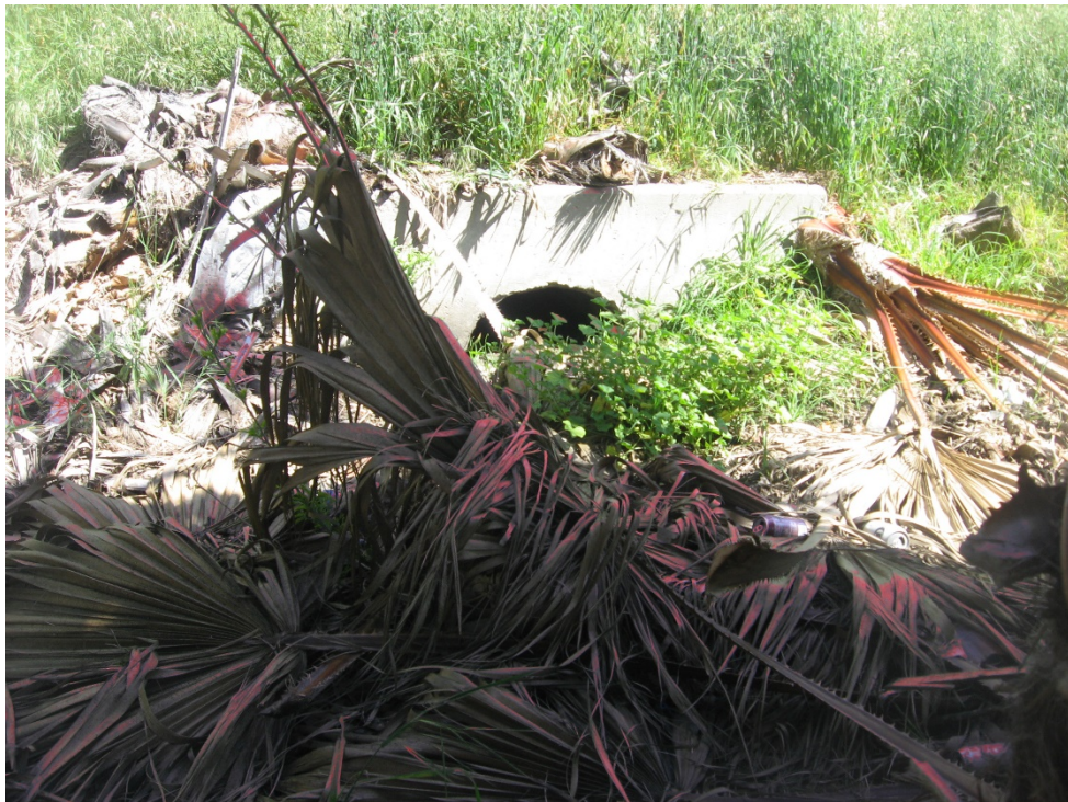
Photograph 6: Culvert outlet from residential neighborhood to the north. No OHWM, bed or bank present (4/21/2020).
