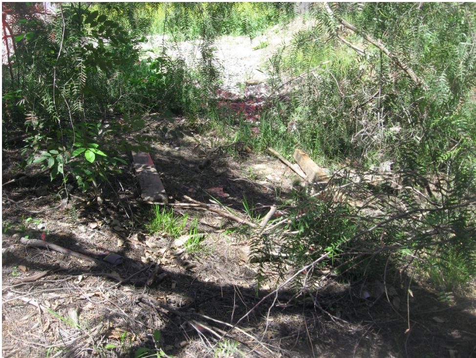
Photograph 12: Existing culvert MP 436.96 passing beneath rail looking upslope (northwest). No OHWM, bed or bank present (4/21/2020).
