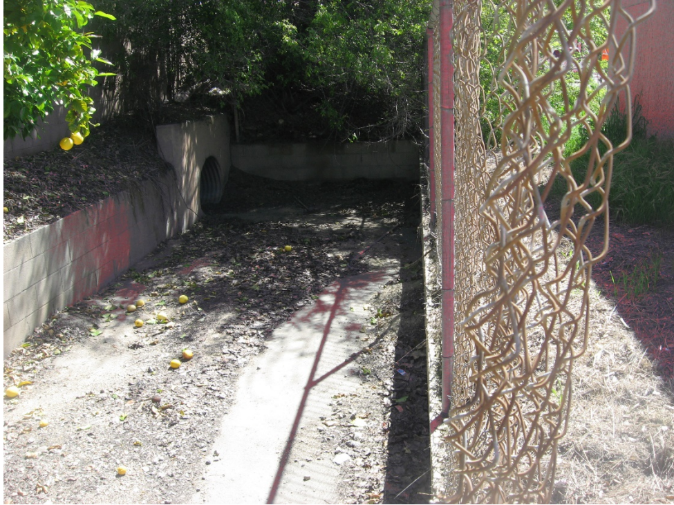
Photograph 1: Off-Site Ditch Constructed in Uplands looking northeast. Ditch drains residential neighborhood to north of Project (4/21/2020).
