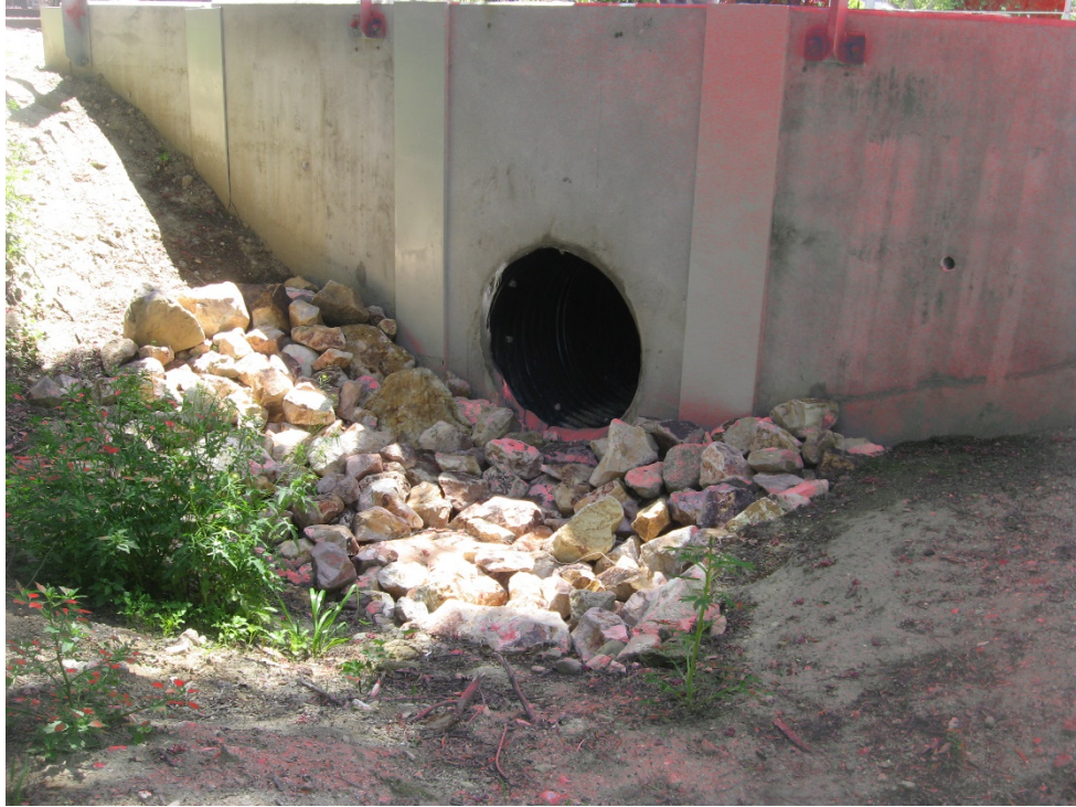
Photograph 13: Inlet of existing culvert MP 436.96 passing beneath the rail looking south. No OHWM, bed or bank present. Based on historic topographic maps, this location did not support a defined drainage (4/21/2020).
