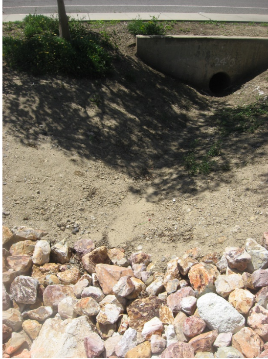
Photograph 15: Swale leading from culvert MP 436.96 to storm drain inlet at Los Angeles Avenue. No OHWM, bed or bank (4/21/2020).
