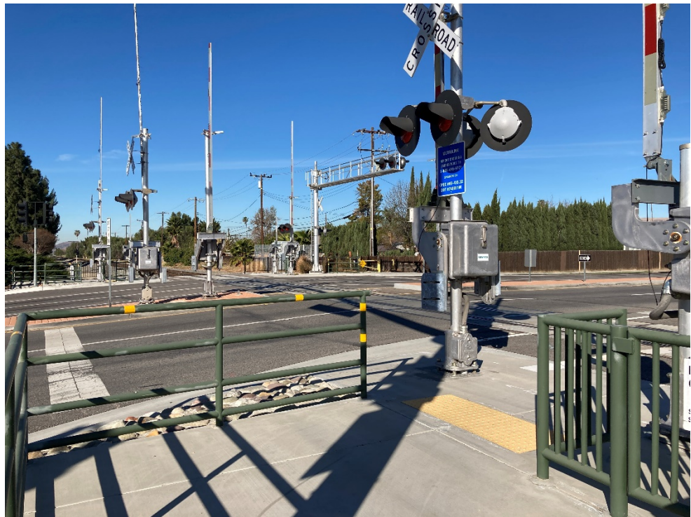
Photo 14: The pedestrian grade crossing at Sycamore Drive was relatively new and included separate gates and signals. The view is to the northwest.
