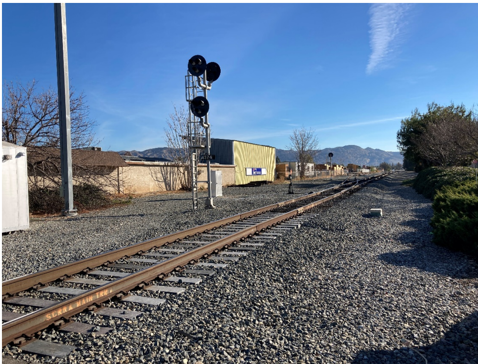
Photo 10: A signal house, signals, and communications tower were located east of the Tapo Street grade crossing. The view is to the east.
