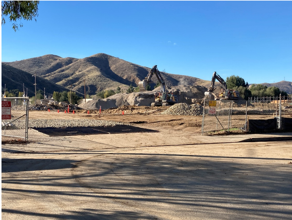
Photo 8: This property located at the eastern extent of Industrial Street was under construction, north of the East Los Angeles Avenue grade crossing. The view is to the south.
