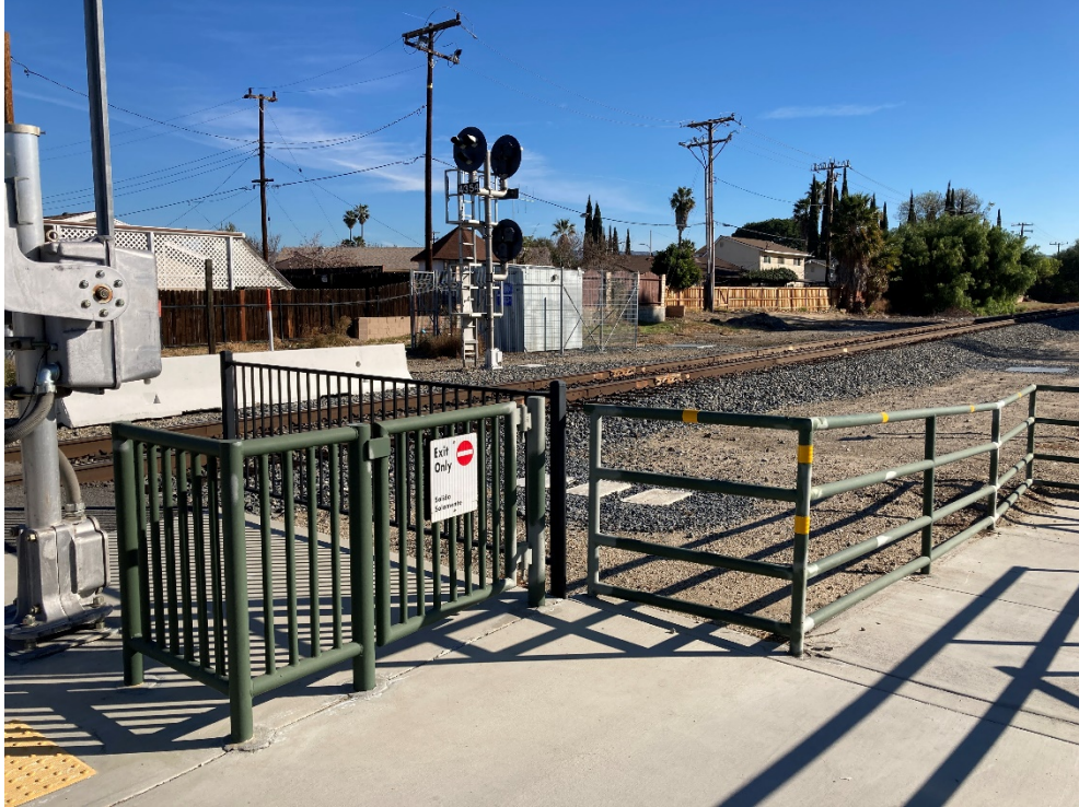
Photo 13: The Sycamore Drive grade crossing included additional signal houses behind security fencing. The view is to the northeast.
