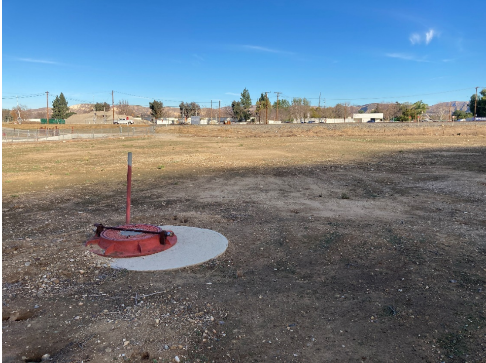
Photo 5: The southern part of the proposed laydown area had a storm drain and remnants of concrete footings. The view is to the north.
